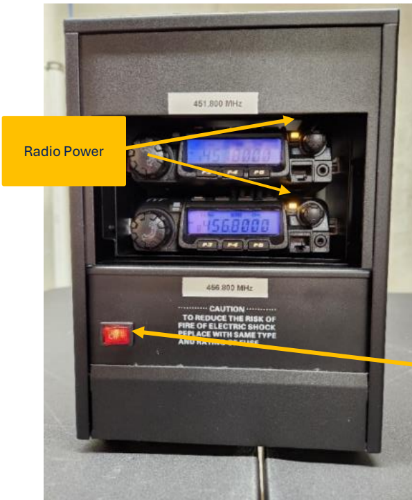
Front view of Repeater Radios
